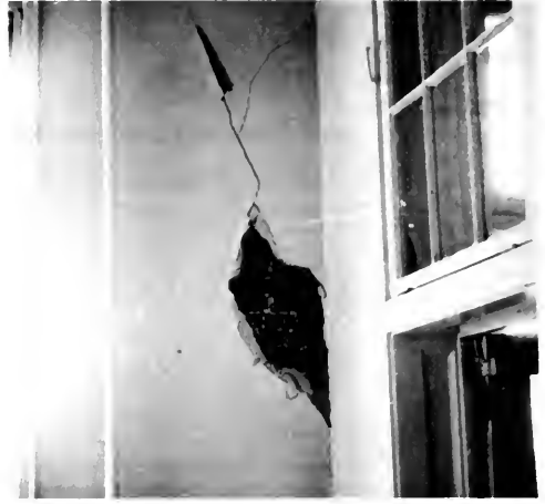
Photo 5. Los Angeles High School. Brick and wall damage at exit door.
